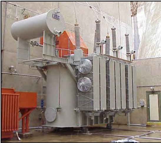
Figure 1 – Typical GSU Three-Phase Transformer.
