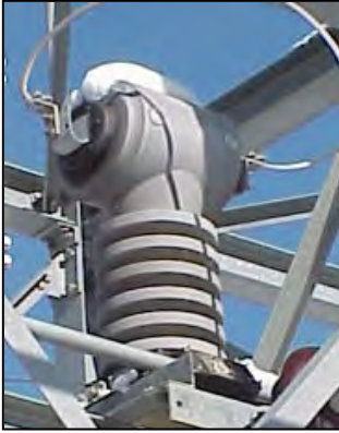
Current Transformer in Switchyard.
