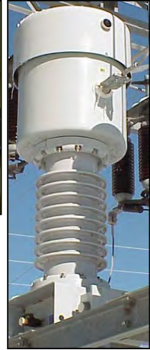
Current Transformer in Switchyard.
